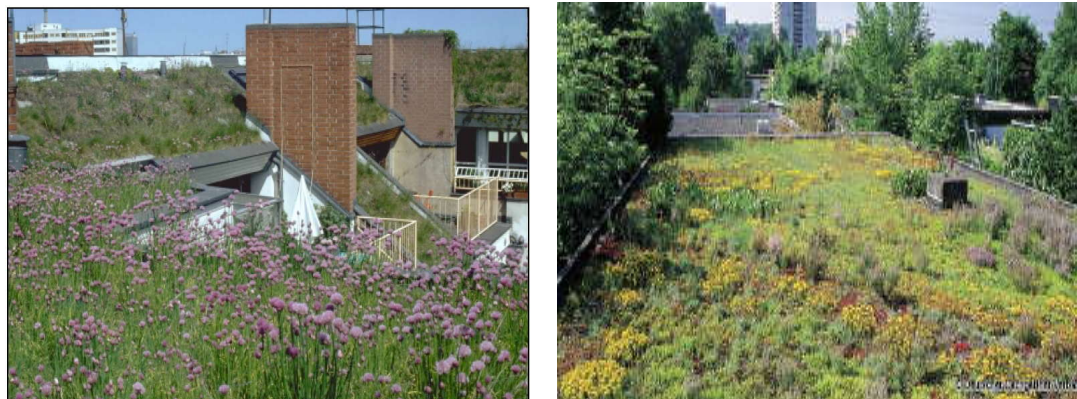
Figure 6-2 Intensive greened roof system established 1984 in Berlin (left) (Sibylle, 2005)
