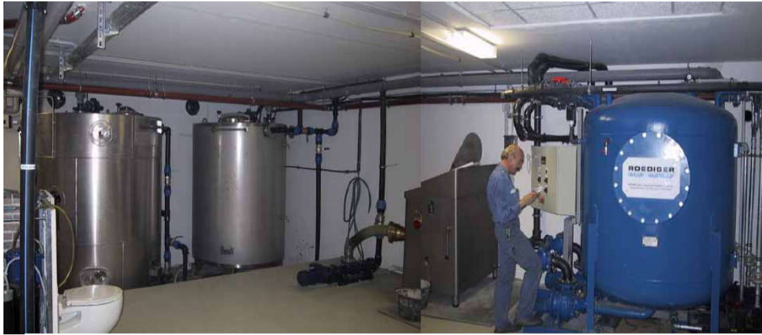
Figure 5-6 Vacuum station, sanitization tank and biogas treatment plant for the collection and anaerobic treatment of black water and bio-waste (Otterpohl, 2001)
