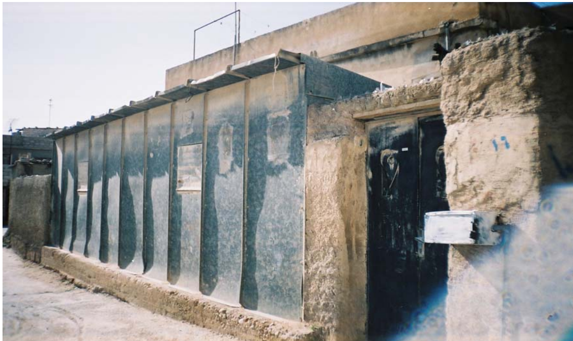
Figure 4.7: Upgrading in Suf camp – little effect on building conditions
