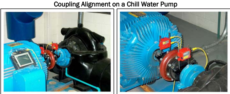
Figure 106 Photos of mounted laser alignment devices on a chill water motor-pump system [WS53]
