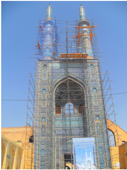
Fig. 7-8: The Jame mosque while being renovated in summer 2010. With minarets as high as 48 meters is a powerful landmark of Yazd. Source: author.
