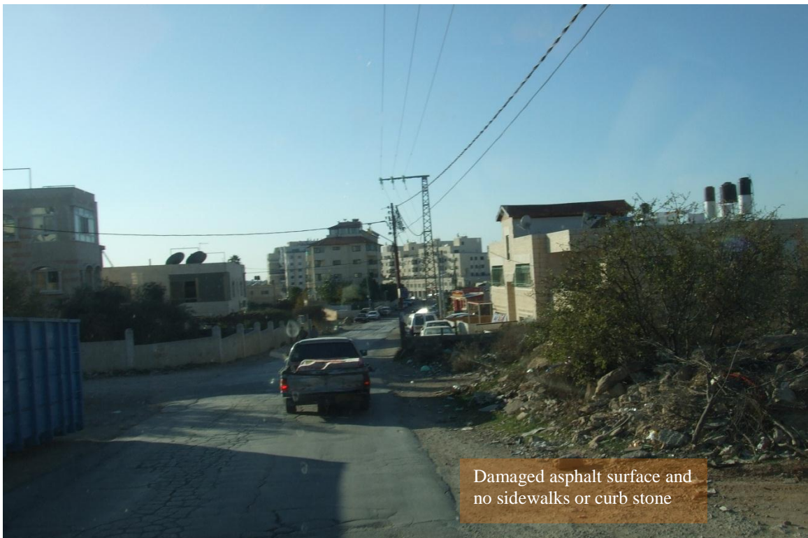
Figure 5.31: Deteriorated infrastructure in Shu'fat Palestinian neighborhood in East Jerusalem, (researcher)
