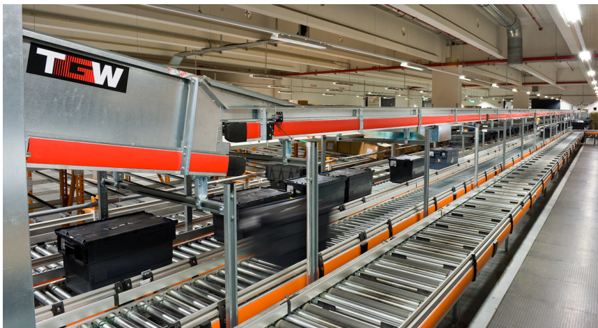
Figure 2.5: Accumulation roller conveyor for the transport of cartons and totes in distribution centers (by Kay-Uwe Rosseburg, available under a Creative Commons Attribution Licence 3.0 at http://commons.wikimedia.org/wiki/File:Accumulation_Roller_Conveyor_for_Cartons_Totes.jpg ).
