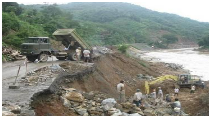
Photo 6.5: Road Eroded by Flood In TTHue
