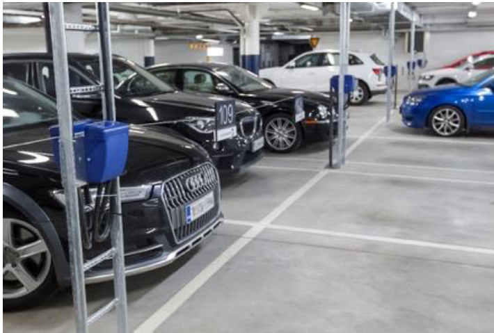
(a) EV ready parking facility
