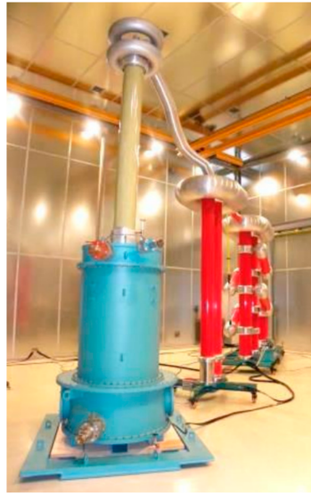
Figure 1. Ester filled HVDC demonstrator in the electrical research Laboratory at Siemens Transformers in Nürnberg, Germany [6].
