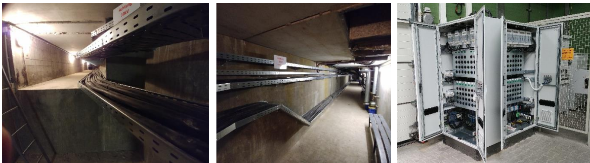
Fig. 5.9: Re-configurable test network available at SGTL – cables installation along the basement of the laboratory area (left-middle) and configuration cabinet for manual network topology implementation (right)
