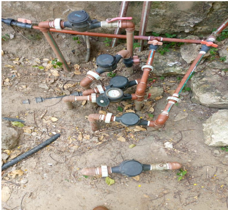
Figure 5.2 Water meters of private network water system
