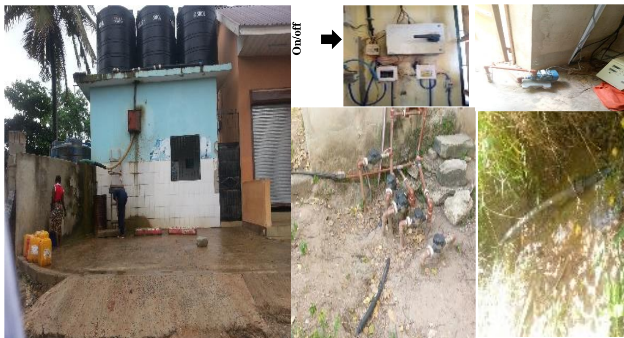
Figure 3.2 Private mechanized boreholes networked water system
