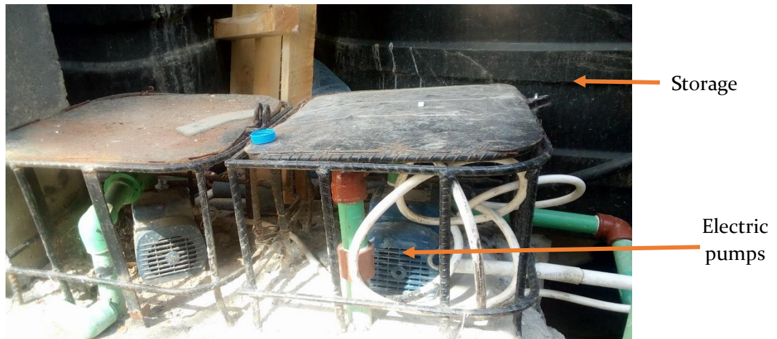
Figure 6.4 Electric pumps for pumping water into storage tanks
