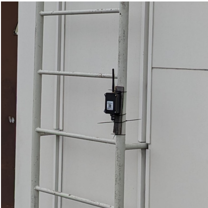
Sensor 3 on the rooftop of the library
