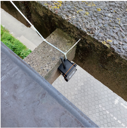
Sensor 1 at the library's west facade
