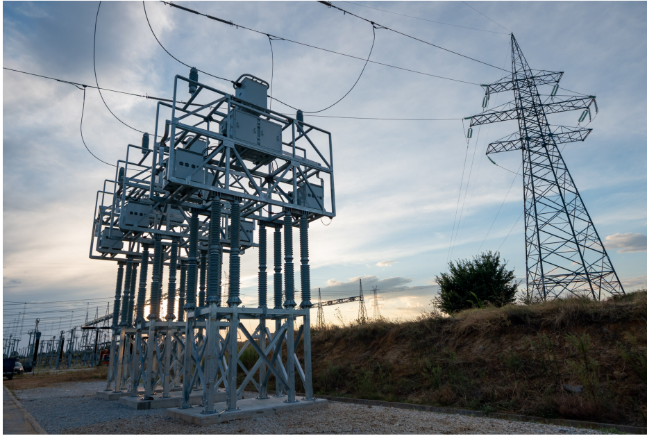
Figure 2.5: Installation of SmartValves at a substation of Greek TSO IPTO ([65])
