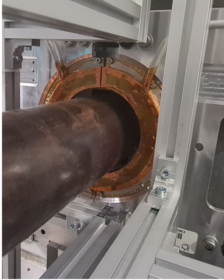
(a) BCM-U station located at the shielding wall of the VELO alcove
