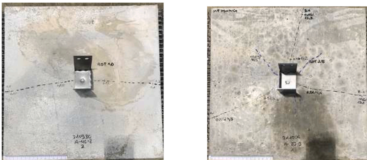
Fig. 9. Crack patterns 1-A (left), 1-B (right).
