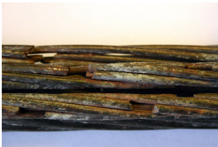
Figure 1: Tension wires broken due to cyclic loadings; Müller, Szugat and Maurer 2016.
