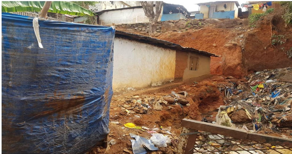
Figure 3. An example of a building exposed to rockfall and mudslide in the event of a heavy downpour and consequential higher soil infiltration. Source: Fieldwork.
