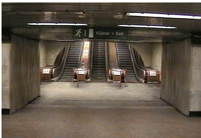
Figure 3 The real escalator
