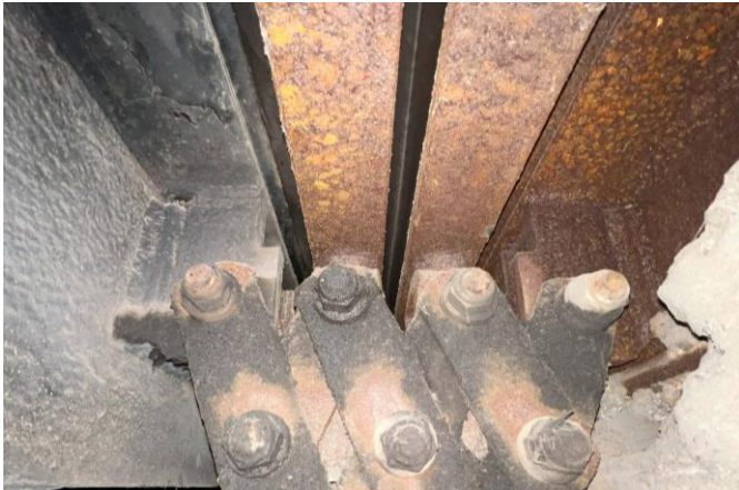
Figure 3 Heavily corroded lamellae and scissor mechanism. Source: Author
