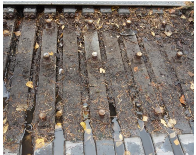
Figure 2 Heavy accumulation of dirt; chipping and flaking of the organic coating. Source: IKS Dresden GmbH
