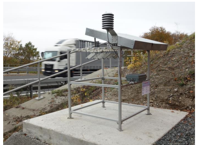
Figure 7 Coils and plates installed on a weather stand. Source: IKS Dresden GmbH
