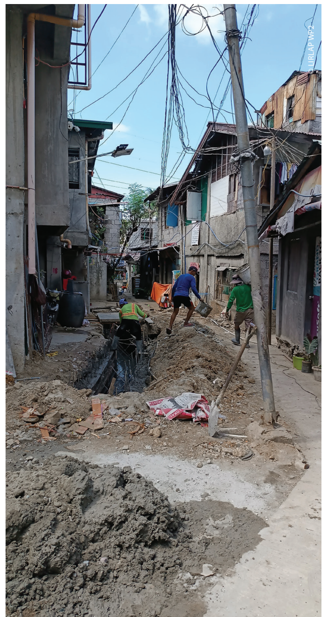
Fig. 11: Needs of reorganizing electrical post in ULHOA due to reblocking. Source: Own Fieldwork in February 2024
