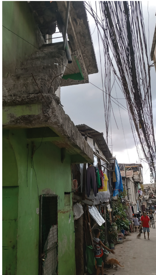
Fig. 10: Partially demolished housing structure in ULHOA due to reblocking. Source: Own fieldwork in February 2024
