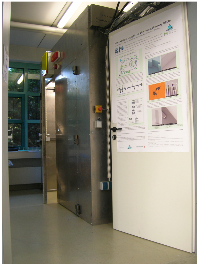
Fig. 4.12.: Exterior view on the experimental hutch build of lead aluminum sandwich plates. The hutch encloses the last beamline section starting at the beryllium window.
