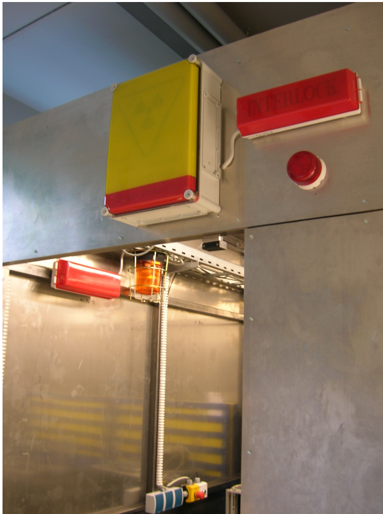
Fig. 4.16.: Warning panels inside and outside the experimental hutch. There is a flashing light and a beamshutter warning panel inside the hutch. The panel restricted area and interlock are installed at the outside of the hutch as well as another flashing light.
