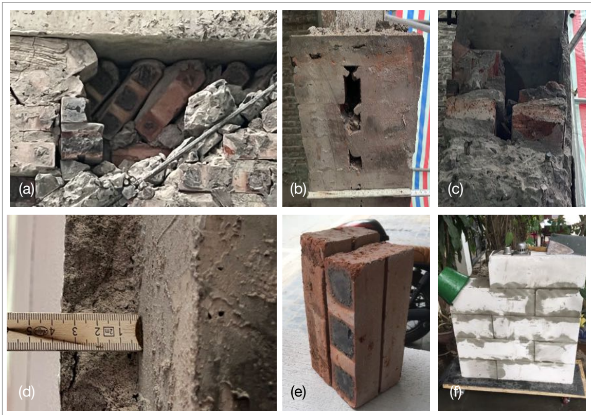
Figure 5.4: (a) Brick Masonry - Transition to Beam, (b) DL Brick cut, Air Gab visible, (c) DL Brick broken, (d) Thickness Plaster Layer, (e) Brick Deviation and (f) AAC Wall Type
