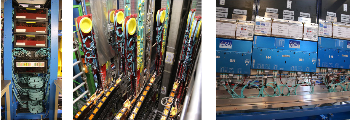
Figure 3.6: Pictures of the bunker patch panel of the C-side (left), the red patch panel directly on the C-Frames (middle) and optical fibres connected to FEBs in the assembly hall (right).
