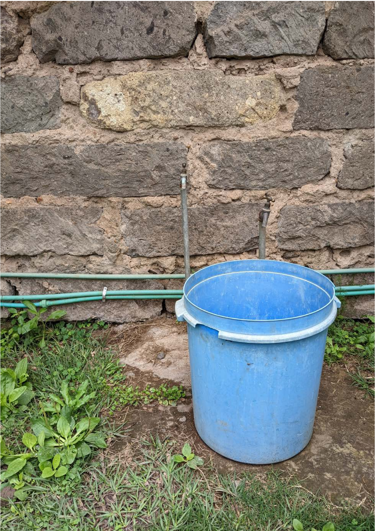
Figure 48: Water taps and bucket in a garden in Ongata Rongai; photo by author (2023).
