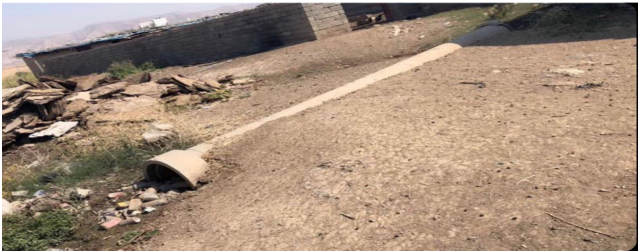
Figure 10- 69: The Destroyed Pipe of the Water Irrigation Project in Expropriated Land in Semel Source: By researcher, 2023
