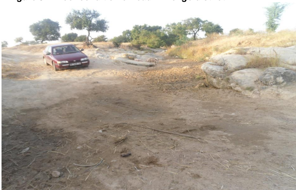
Figure 3.7: Poor condition of road in Bongo district
