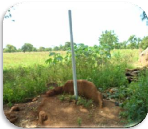
Figure 7.12: Collapsed Sanitary Facility in Damdo
