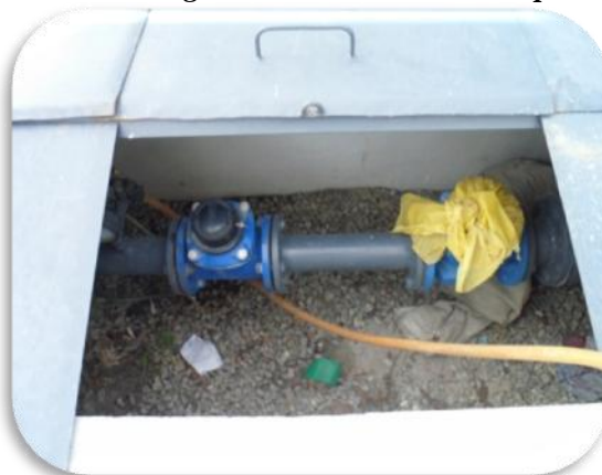
Figure 7.5: Underground Connection in Buipe
