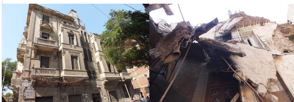
Figure 11-6 Registered Building, intentionally demolished core, 51 al-Qabwa St. Misr al-Qadima Source (NOUH, 2011)
