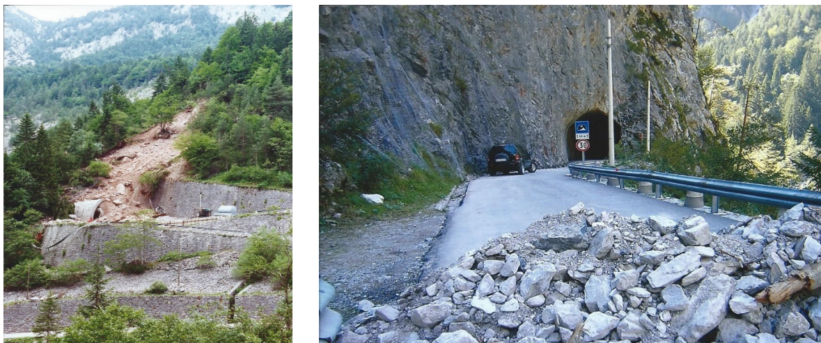
Figure 23 Left: Landslide in the Fella River Catchment; Right: Rock fall in the Fella River Catchment (Photos: Courtesy of Armando Coianiz)
