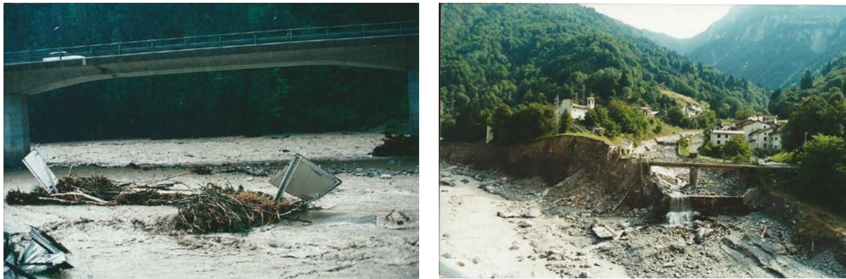
Figure 33 Flash flood and debris flow event that occurred in the Italian case study area in August 2003. Left: Traces of debris; Right: Erosion and destroyed house along the river bed (Source: Courtesy of Armando Coianiz)
