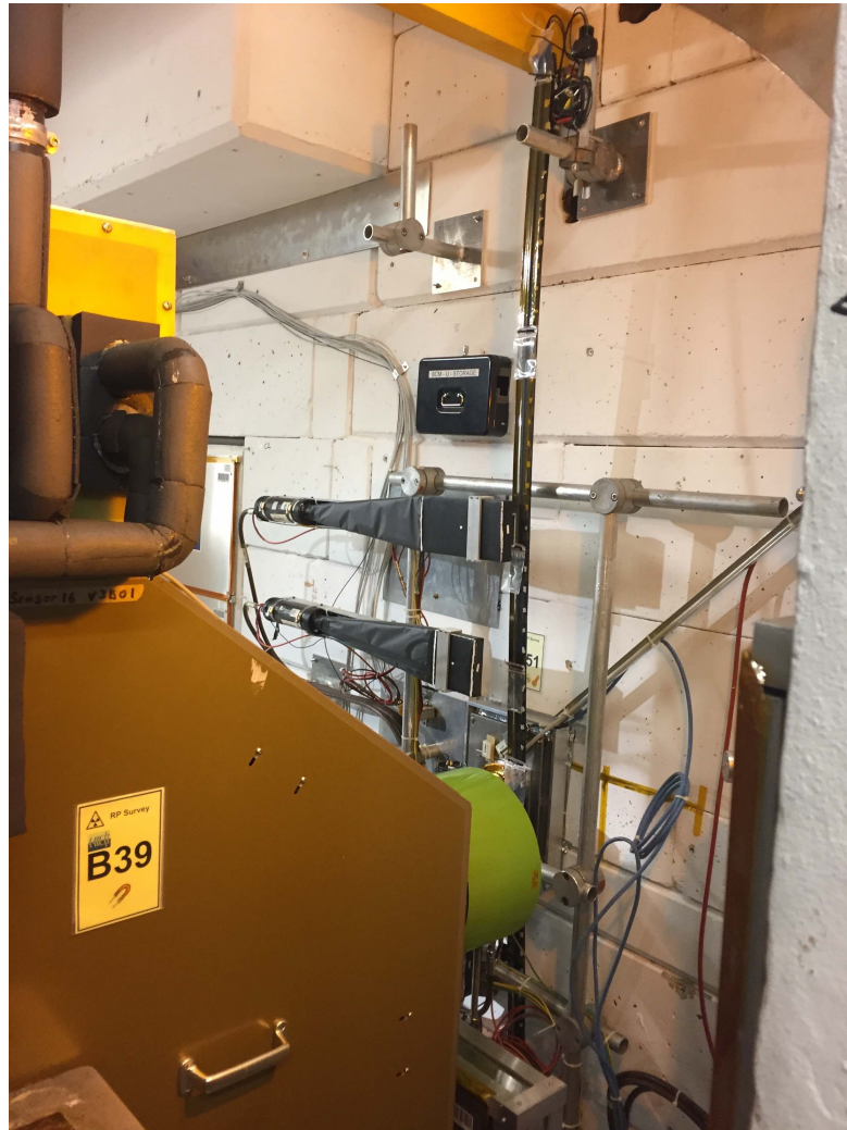
Fig. A.2.: Fibre module installed in the LHCb cavern at the shielding wall near the VELO.
