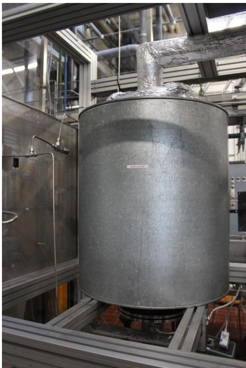
Figure 48: The electrical preheater of the inflowing gas stream
